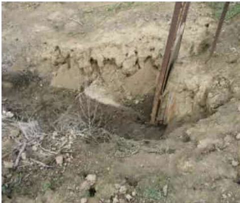
11/27/2012 (ST0003U01 LM:18.612) : WS view: sloughing at outlet pipe
