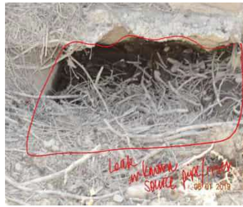
11/12/2019 (ST0003U01 LM:12.963) : WS view: leak visible on WS.
