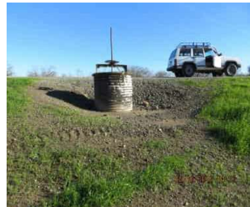
12/10/2012 (ST0003U01 LM:12.963) : WS view: soil erosion around CMP riser
