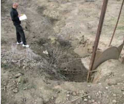
11/27/2012 (ST0003U01 LM:18.612) : WS view: damaged levee slope
