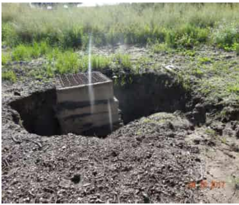
04/20/2017 (ST0003U01 LM:12.963) : Erosion hole at WS surge box 4/20/2017
