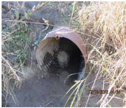
12/10/2012 (ST0003U01 LM:12.963) : LS view: outlet pipe on water transfer ditch
