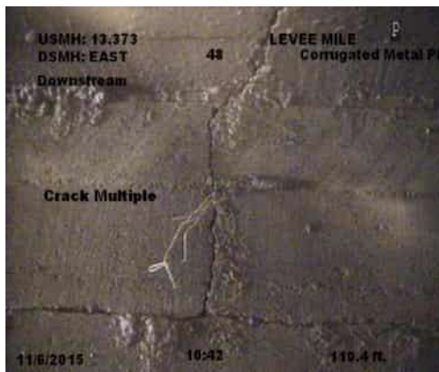
06/16/2016 (ST0003U01 LM:13.376) : Snapshot from internal inspection performed by Nor-Cal Pipeline Services on 11/6/2015.
