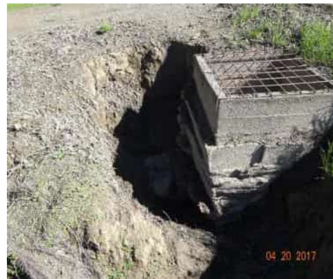
04/20/2017 (ST0003U01 LM:12.963) : Erosion hole at WS surge box 4/20/2017
