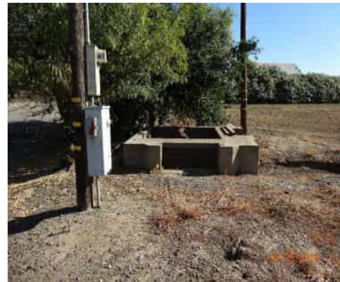
08/05/2019 (ST0003U01 LM:18.612) : LS view: power meter and concrete structure located on the LS.
