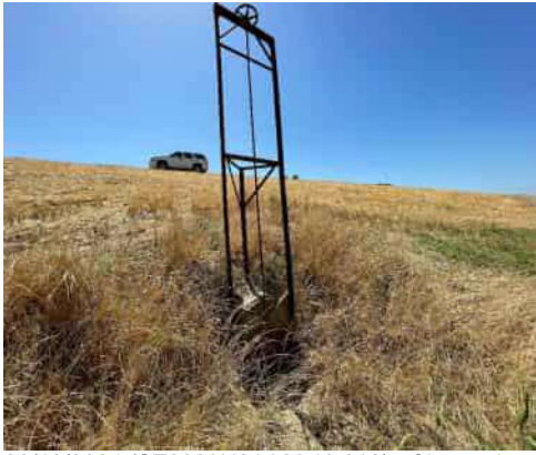
06/13/2024 (ST0003U01 LM:18.612) : Closer view of slide gate on WS
