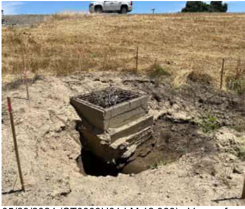
05/29/2024 (ST0003U01 LM:12.963) : Veew of severe erosion at concrete box
