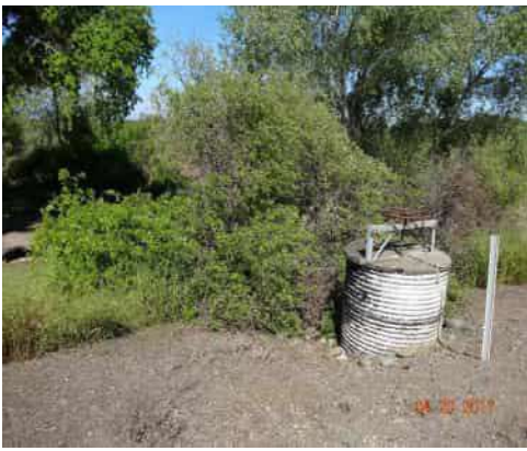
04/20/2017 (ST0003U01 LM:13.376) : Fallen oak tree over WS pipe end
