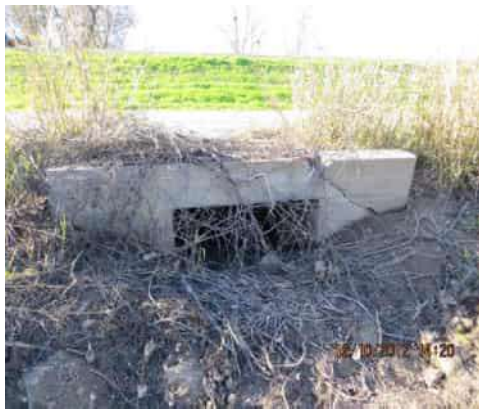
12/10/2012 (ST0003U01 LM:13.376) : LS view: damaged concrete culvert across the road
