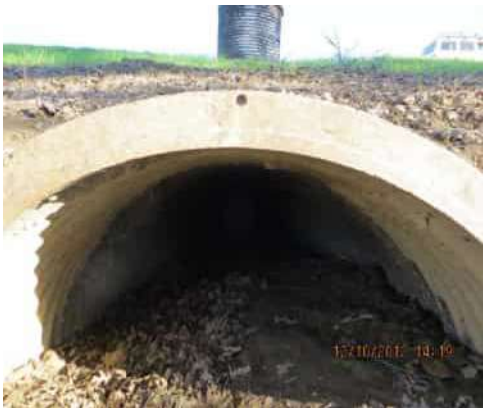
12/10/2012 (ST0003U01 LM:13.376) : WS view: silted concrete lined CMP outlet pipe
