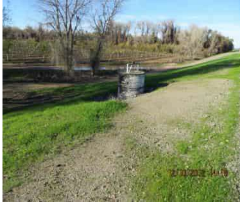
12/10/2012 (ST0003U01 LM:13.376) : WS view: CMP riser with slide gate
