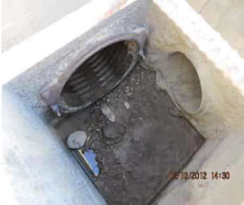
12/10/2012 (ST0003U01 LM:12.963) : WS view: CMP in surge box. Flap gate missing.
