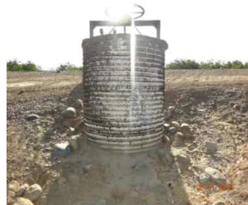
08/01/2019 (ST0003U01 LM:13.376) : WS view: CMP riser with slide gate.
