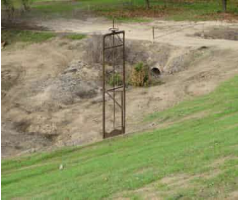
11/27/2012 (ST0003U01 LM:18.612) : WS view: overview of sliding gate structure
