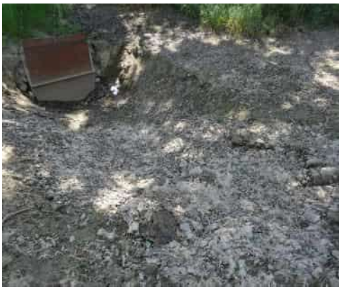
04/14/2016 (ST0003U01 LM:13.376) : WS slope: sediment buildup temporarily prevented from entering WS pipe outlet by wooden board.
