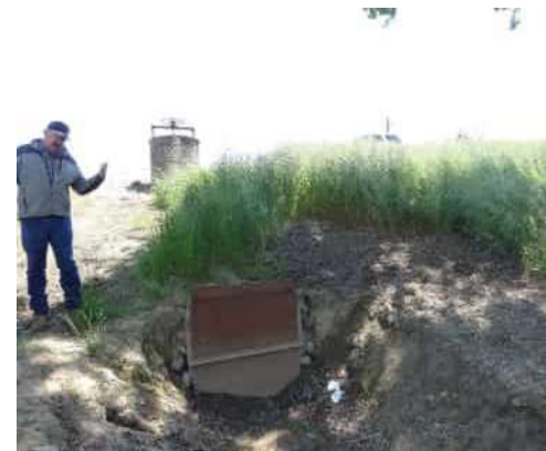
04/14/2016 (ST0003U01 LM:13.376) : View up WS slope: sediment buildup against board covering pipe outlet. Board placed as a temporary fix.
