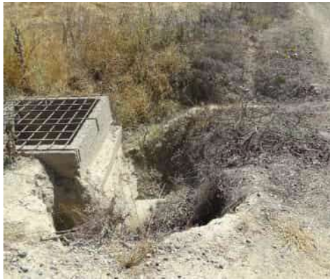
08/30/2018 (ST0003U01 LM:12.963) : WS view: same massive erosion around concrete surge box.
