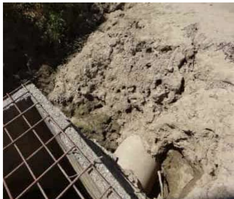
04/14/2016 (ST0003U01 LM:12.963) : WS slope: another view of scour hole
