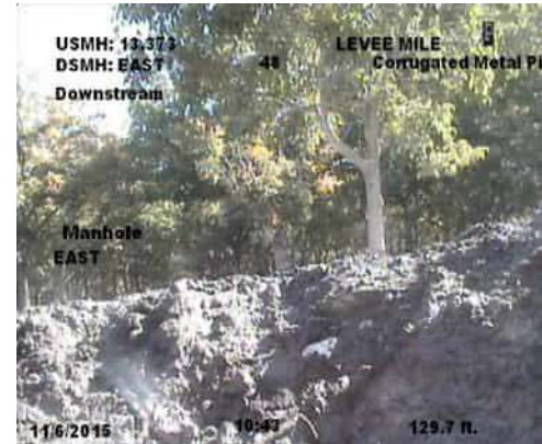
06/16/2016 (ST0003U01 LM:13.376) : Snapshot from internal inspection performed by Nor-Cal Pipeline Services on 11/6/2015.
