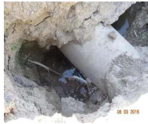
06/03/2016 (ST0003U01 LM:12.963) : WS slope: close-up view of scour hole at WS slope.
