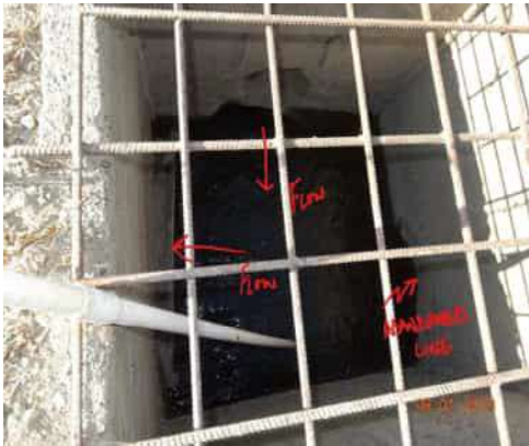
08/01/2019 (ST0003U01 LM:12.963) : WS view: pipe running during inspection (flow schematics).
