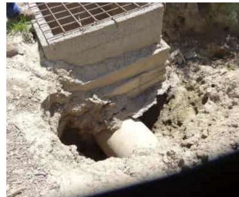
04/14/2016 (ST0003U01 LM:12.963) : WS slope: Massive erosion and scour hole on two sides of concrete surge box. Pipe exposed.
