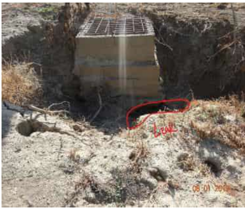
11/12/2019 (ST0003U01 LM:12.963) : WS view: erosion associated with concrete box.
