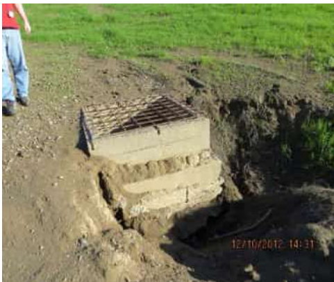
12/10/2012 (ST0003U01 LM:12.963) : WS view: huge erosion around concrete surge box
