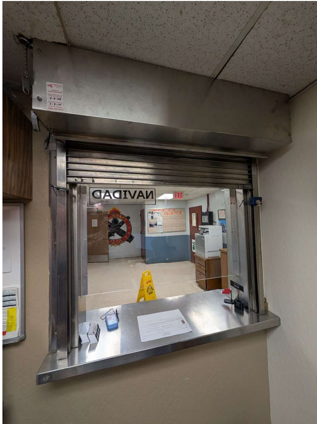
Photo C-1: Existing counter fire door assembly (door held open with temporary field bolt; counterbalance springs inoperative)
