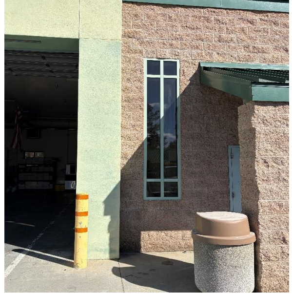
Equipment shop_2 (one window)
