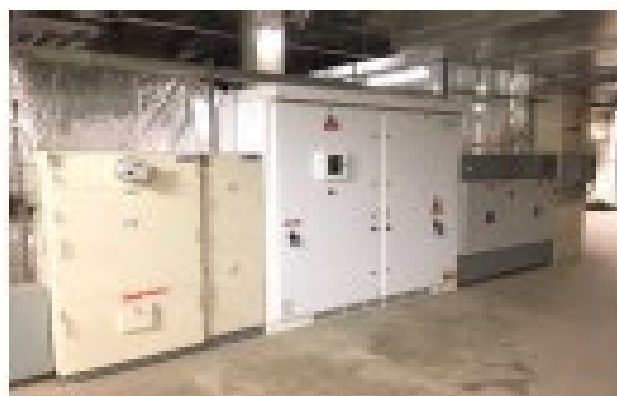
Sheet A6 Bldg East 7 th Floor Penthouse Solar Inverter "A"
