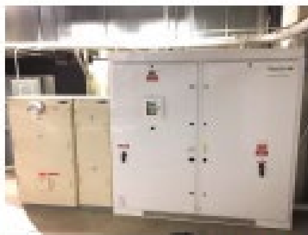
Sheet A7 Bldg East 7 th Floor Penthouse Solar Inverter "B"
